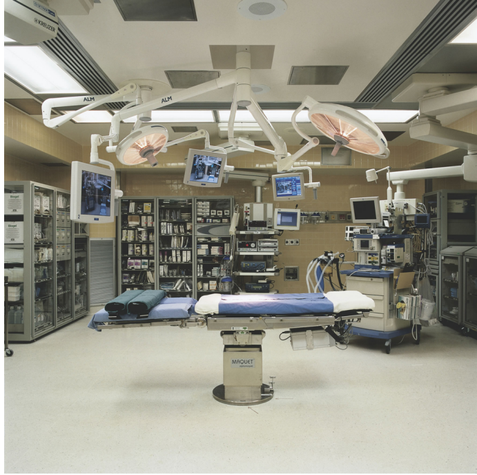
Figure 1-1: The Operating Room of the Future at MGH
